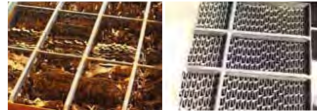
Regular steel used (serious corrosion shown)
