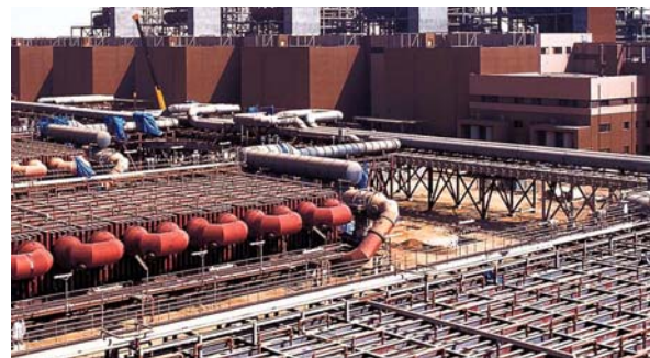
Desalination Plant (Resource : Doo San heavy industries)
